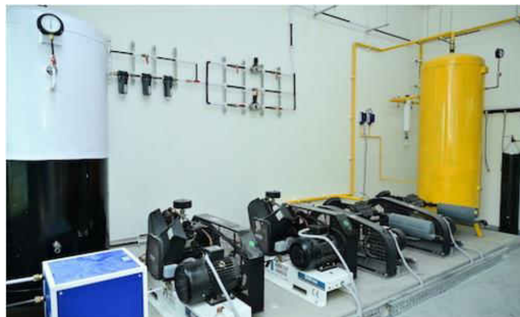
UTILITY GAS PIPING
